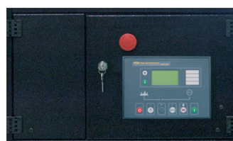
Deep Sea 7210 Control Panel
